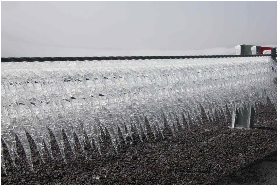
A storm on March 29, 2005 left ice frozen to the guard rails along the summit roads. Picture taken on March 30, 2005.
